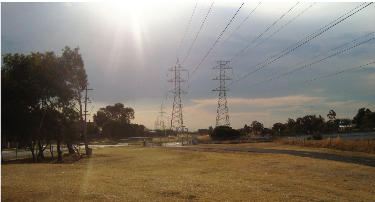
Figure 9: Electricity pylons during a heatwave; extreme heat puts increasing pressure on infrastructure.
